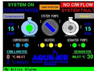
PLC / Touchscreen Chiller Controls with Remote System Monitoring
